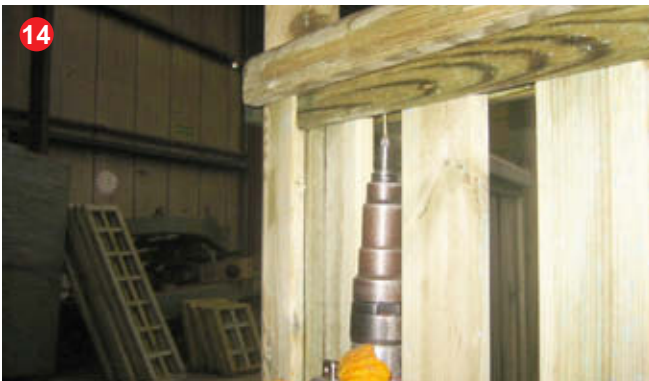
14 Secure hand rails by screwing through fence into handrail using 3 x 40mm screws.
